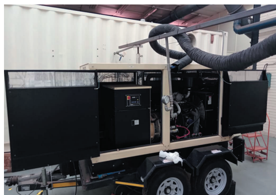
Figure 4: Externally Coupled Mobile Generator
